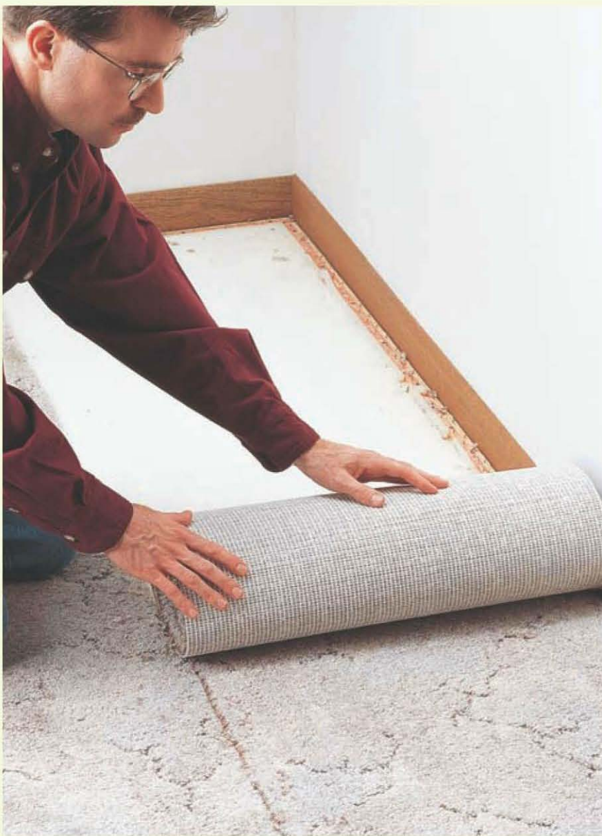
Tacked carpet: Cut wall-to-wall carpeting into strips as you work to make removal and disposal easier.
