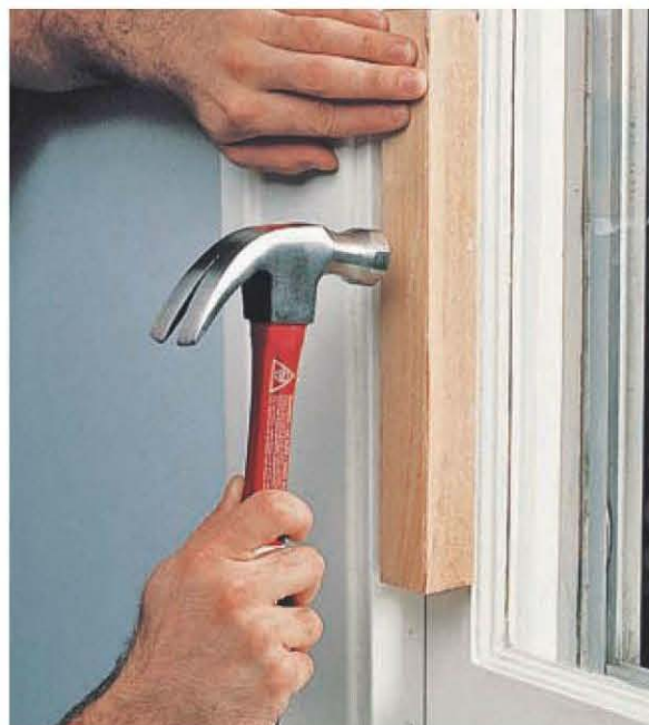
Stubborn windows may require a little persuasion to unstuck. After cutting paint seals, tap (carefully) along the sash frame with a hammer and wood block.
