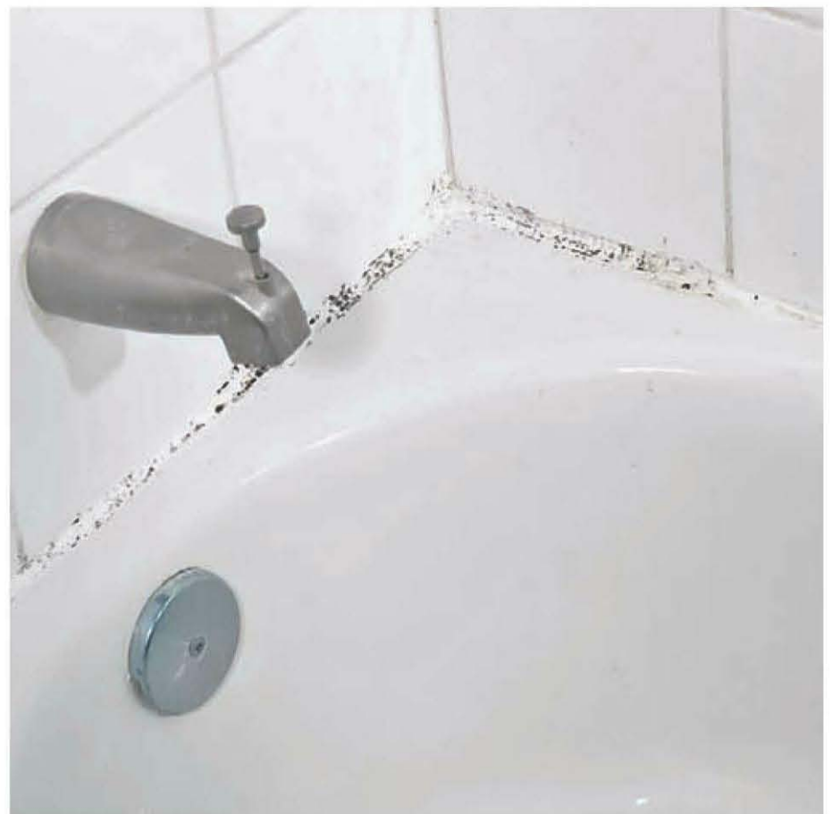
Just about any tub or shower can benefit from a thorough cleaning and re-caulking of its seams.
