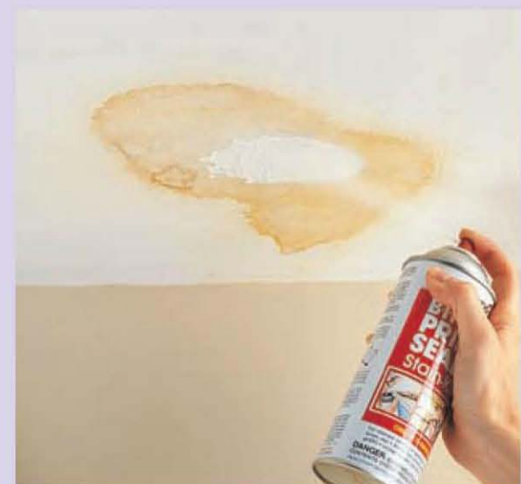
Water or rust stains may indicate water damage. Check for leaking pipes and soft plaster, make needed repairs, then seal the area with stain-killing sealer.
