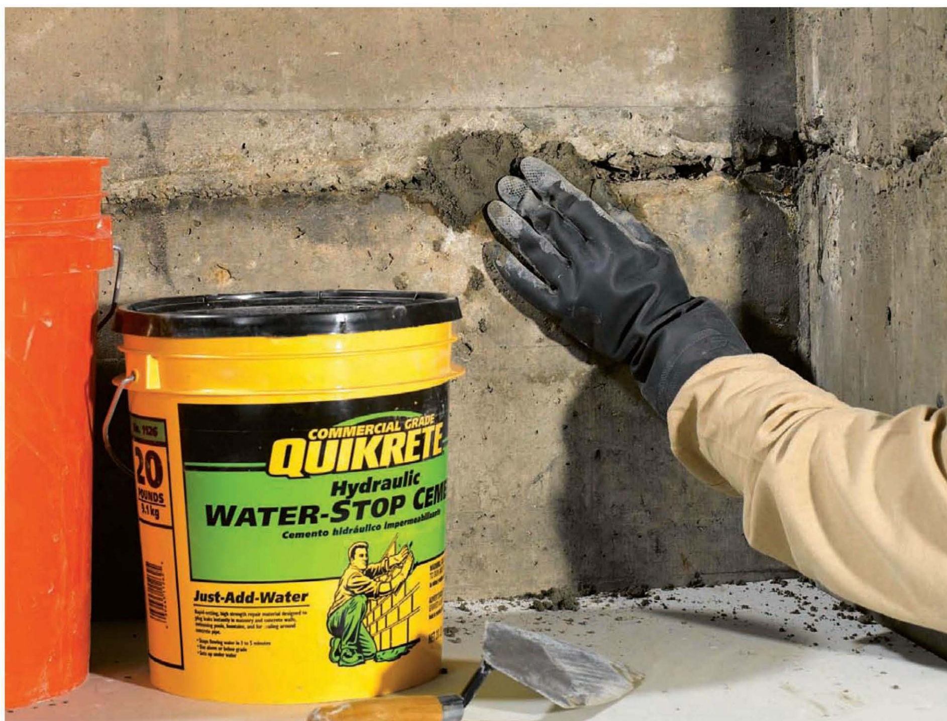
Hydraulic cement expands as it dries, creating a watertight seal. Repairs can be left as-is or be covered with masonry paint or waterproofer.
