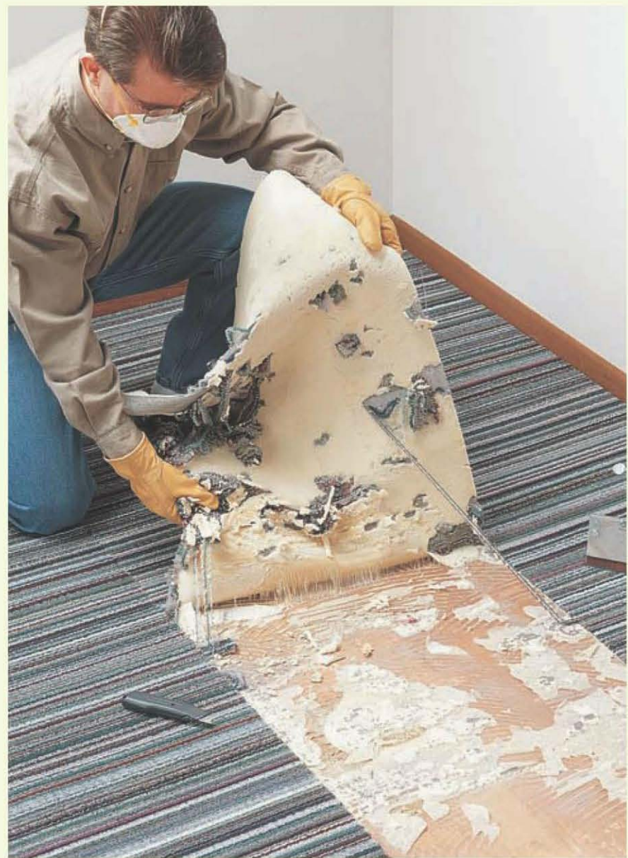
Bonded carpet: Carpet that has been bonded to the floor or floor underlayment is a pain to remove. You may be better off removing and replacing underlayment rather than trying to salvage it.
