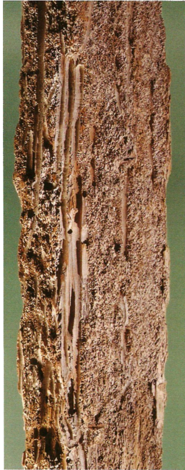
Figure 2.43 • Wood damaged by marine borers. (Photo by Randy O'Rourke)
