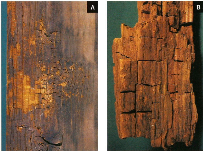
Figure 2.45 • Infection with brown rot (A) eventually results in cubical breakup of the wood (B). (Photos by Randy O'Rourke)
