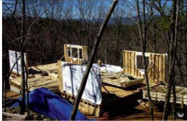
Figure 12.21 Moving on, we can see the walls are erecting quickly. With only two workers, four walls are now in place.
