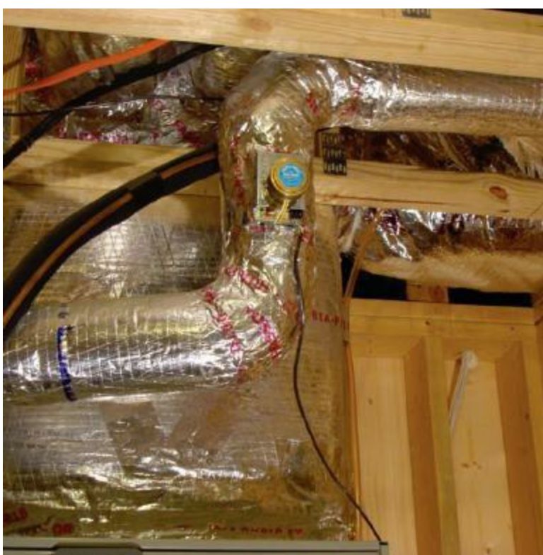
Figure 6.18 Fresh air intake damper.
