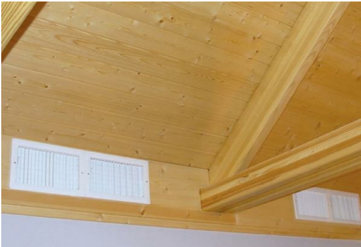
Figure 12.35 Upper return vents.
