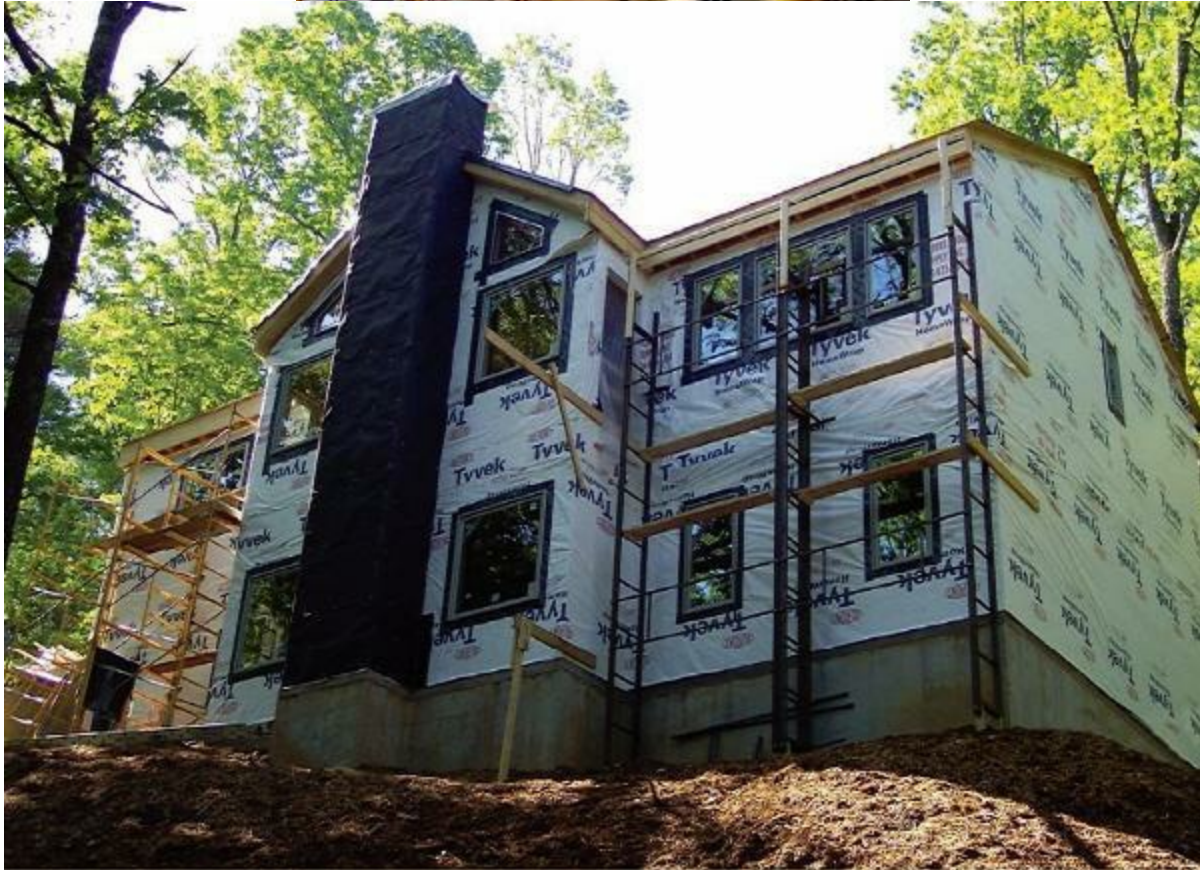
Figure 12.31 The ice/watershield membrane sealing strips are visible around the window perimeter as well as entire building envelope's wrapping (TYVEK).
