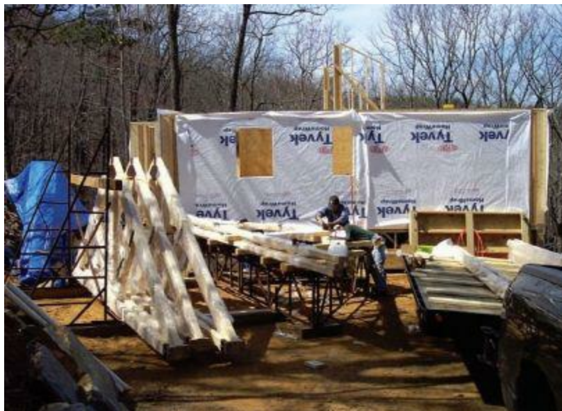
Figure 12.25 Before the boom truck is scheduled we need to assemble the Timber Trusses at the
