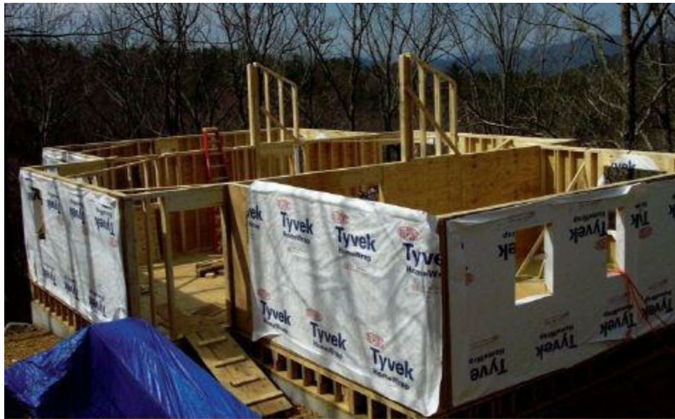
Figure 12.24 And finally, all the major walls, without the top gable sections, are erected and waiting for the boom truck and the Timber Trusses.
