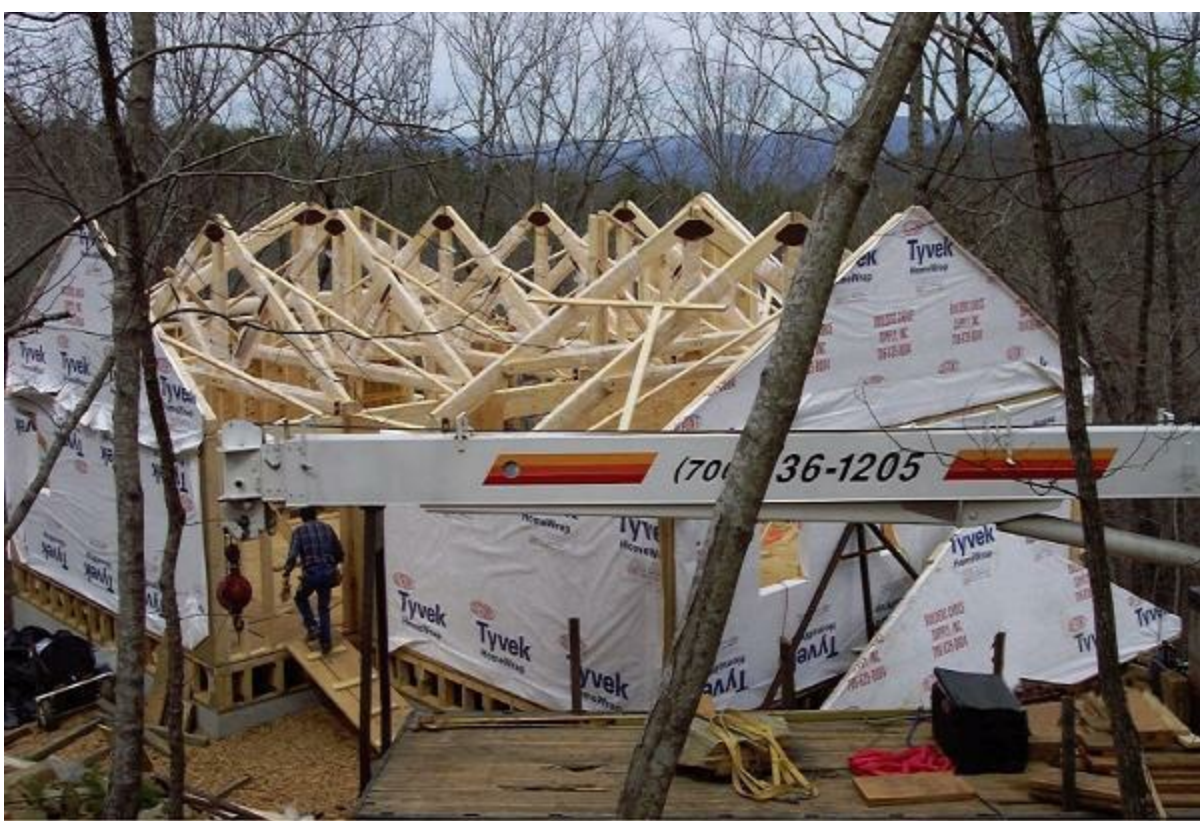
Figure 12.28 Near the end of the boom-truck-lifting day, most of the Timber Trusses are in place. Several hours of boom truck time, even on this tight mountain site, facilitated the erecting of the nine Timber Trusses and the four main Gable modules.
