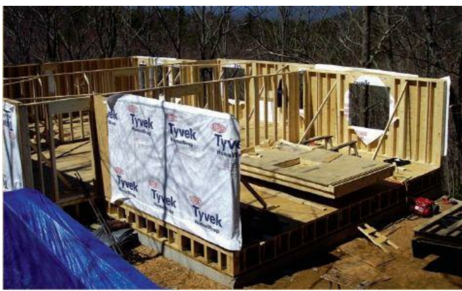
Figure 12.23 The few interior walls (for the great room with Timber Truss support) are filling in the main floor structure.
