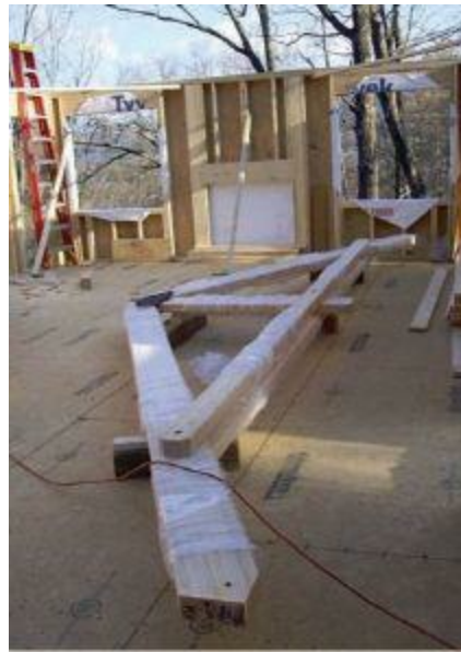
Figure 12.26 One of the King 6/12-26 foot bedroom wing Timber Trusses on the floor ready to be lifted by the boom truck.
