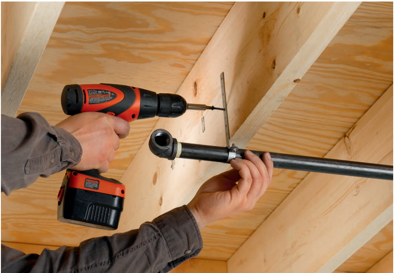
Running new pipe lines allows you to enjoy the practical and cost-savings benefits of natural gas in all areas of your home.
