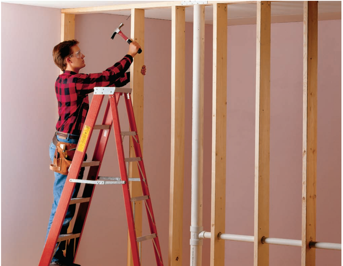
Use 2 × 6 studs to frame “wet walls” when constructing a new bathroom or kitchen. Thicker walls provide more room to run drain pipes and main waste-vent stacks, making installation much easier.
