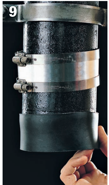
9 Make sure the cast-iron pipe is seated snugly against the rubber separator ring molded into the interior of the sleeve.
