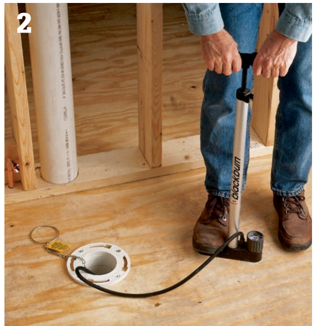
Block toilet drains with a test balloon designed for a closet bend. Large test balloons may have to be inflated with an air pump.
