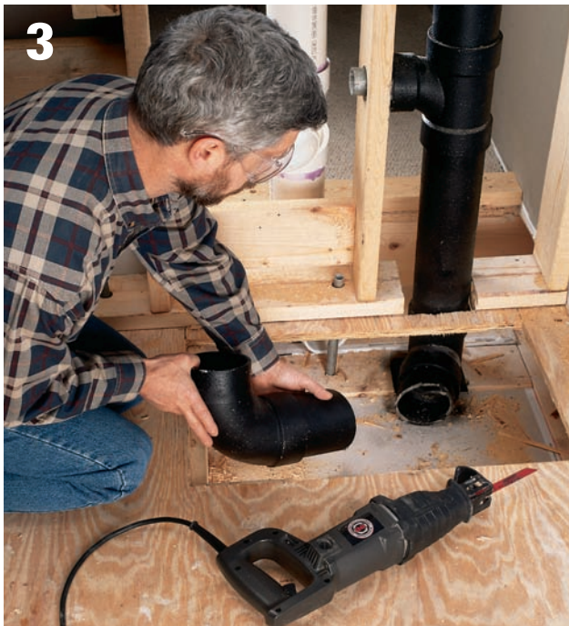
3 Cut away the old closet bend as close as possible to the old waste-vent stack, cutting first with a grinder equipped with a metal-cutting blade, then finishing with a reciprocating saw.
