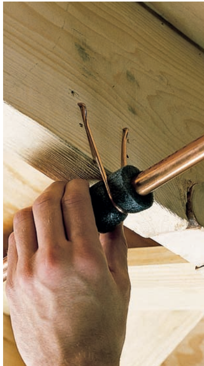
Loose pipes may bang or rub against joist hangers, creating noise. Use pieces of foam rubber pipe insulation to cushion pipes.
