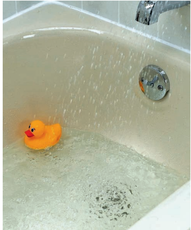
As with bathroom sinks, tub and shower drain pipes may become clogged with soap and hair. The drain stopping mechanisms can also require cleaning and adjustment.
