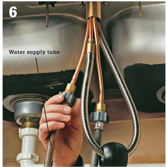
6 Hook up the water supply tubes to the faucet inlets. Make sure the tubes are long enough to reach the supply risers without stretching or kinking.
