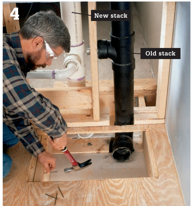
4 If a joist obstructs the route to a new waste-vent stack, cut away a section of the floor joist. Install double headers and metal joist hangers to support the ends of the cut joist.
