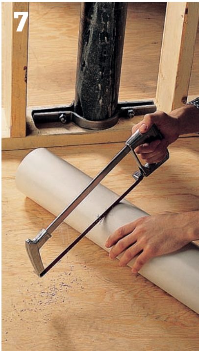
7 Cut a length of PVC plastic pipe to be \frac{1}{2} " shorter than the section of cast-iron pipe that has been cut away.
