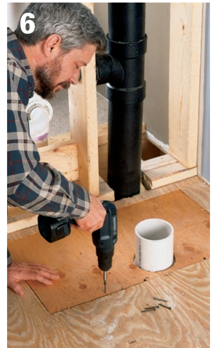
6 Cut a piece of exterior-grade plywood to fit the cutout floor area, and use a jigsaw to cut an opening for the toilet drain stub-out. Position the plywood, and attach it to joists and blocking with 2" screws.
