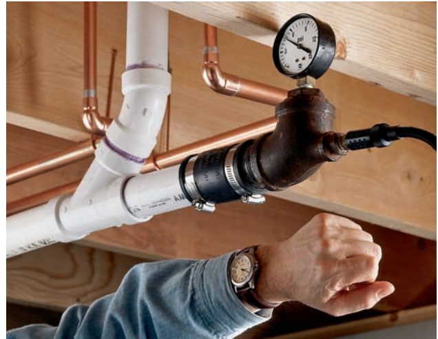
A pressure gauge and air pump are used to test DWV lines. The system is first blocked off at each fixture and at points near where the new drain and vent pipes connect to the main stack. Air is then pumped into the system to a pressure of 5 pounds per square inch (psi). To pass inspection, the system must hold this pressure for 15 minutes.
