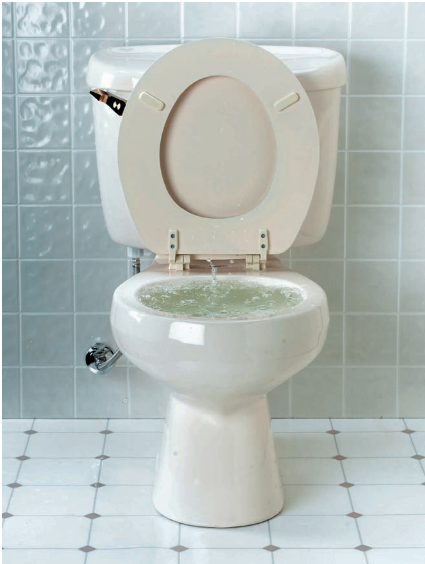
A blockage in the toilet bowl leaves flush water from the tank nowhere to go but on the floor.
