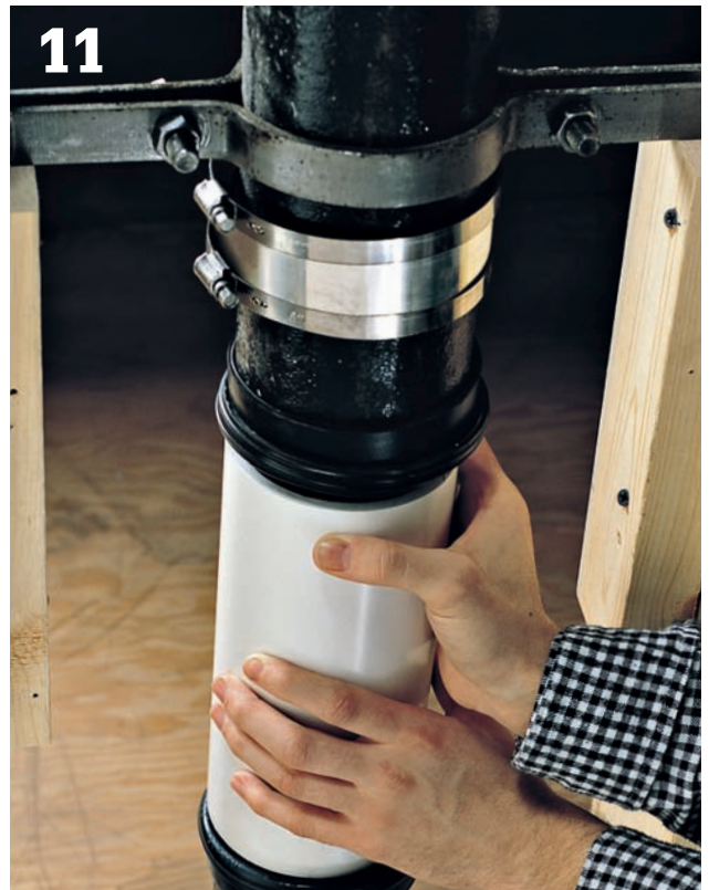
11 Position the new plastic pipe so it is aligned with the cast-iron pipes.
