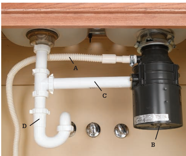
In this arrangement, the dishwasher drain hose (A) attaches to the food disposer (B), and a trap arm (C) leads from the disposer to the P-trap (D).
