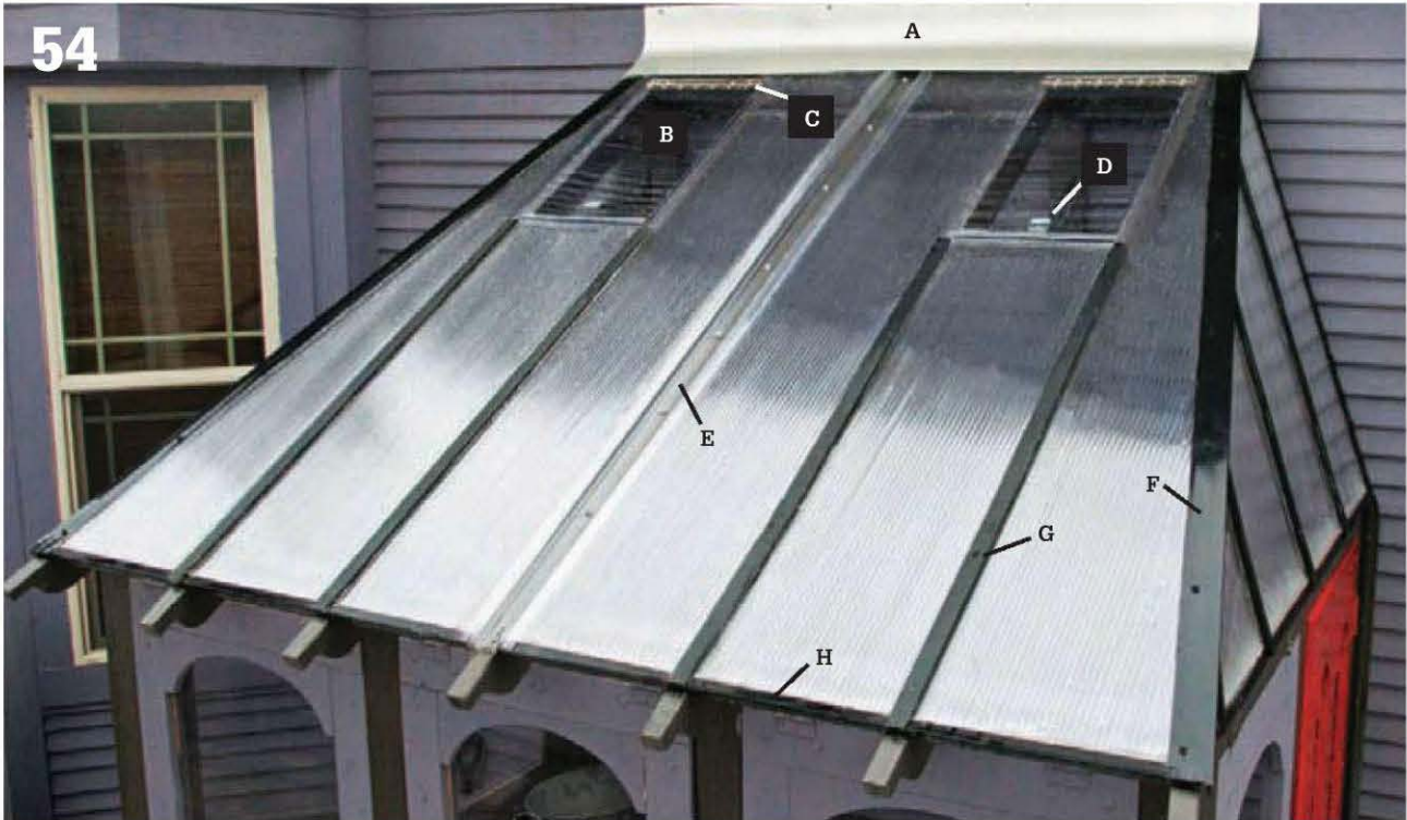
Add trim elements to complete the roof. Parts of the roof trim system include: Flashing over ridge (A); Clear vent panel (B) attached with piano hinge (C) and automatic closer (D); Seaming strip (E); Metal drip cap for edges (F); ¼ x 1½" wood battens at rafter locations (G); vinyl cap molding at eave edges (H).
