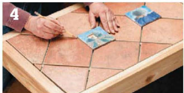
4 Dry-fit the field tiles using tile spacers to set consistent gaps. Set the accent tiles in place and mark the field tiles for cutting.
