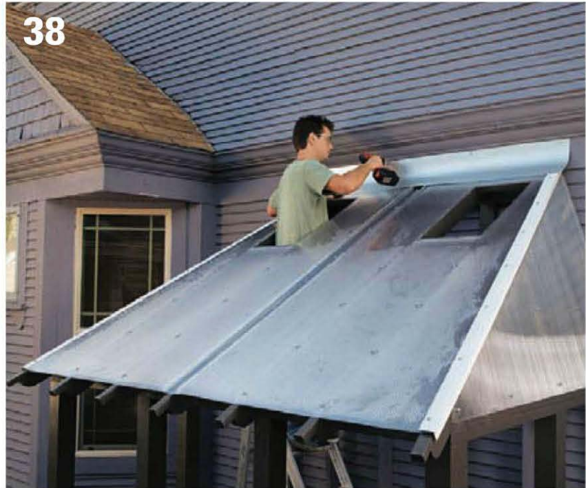
38 Cover the gap between the standalone greenhouse structure and the house with metal flashing. Aluminum handy flashing (12" width) can be fastened to the house and lightly creased so it extends over the gap and forms a seal without any physical connection to the greenhouse.
