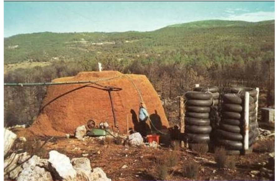
Gas and hot water production system
