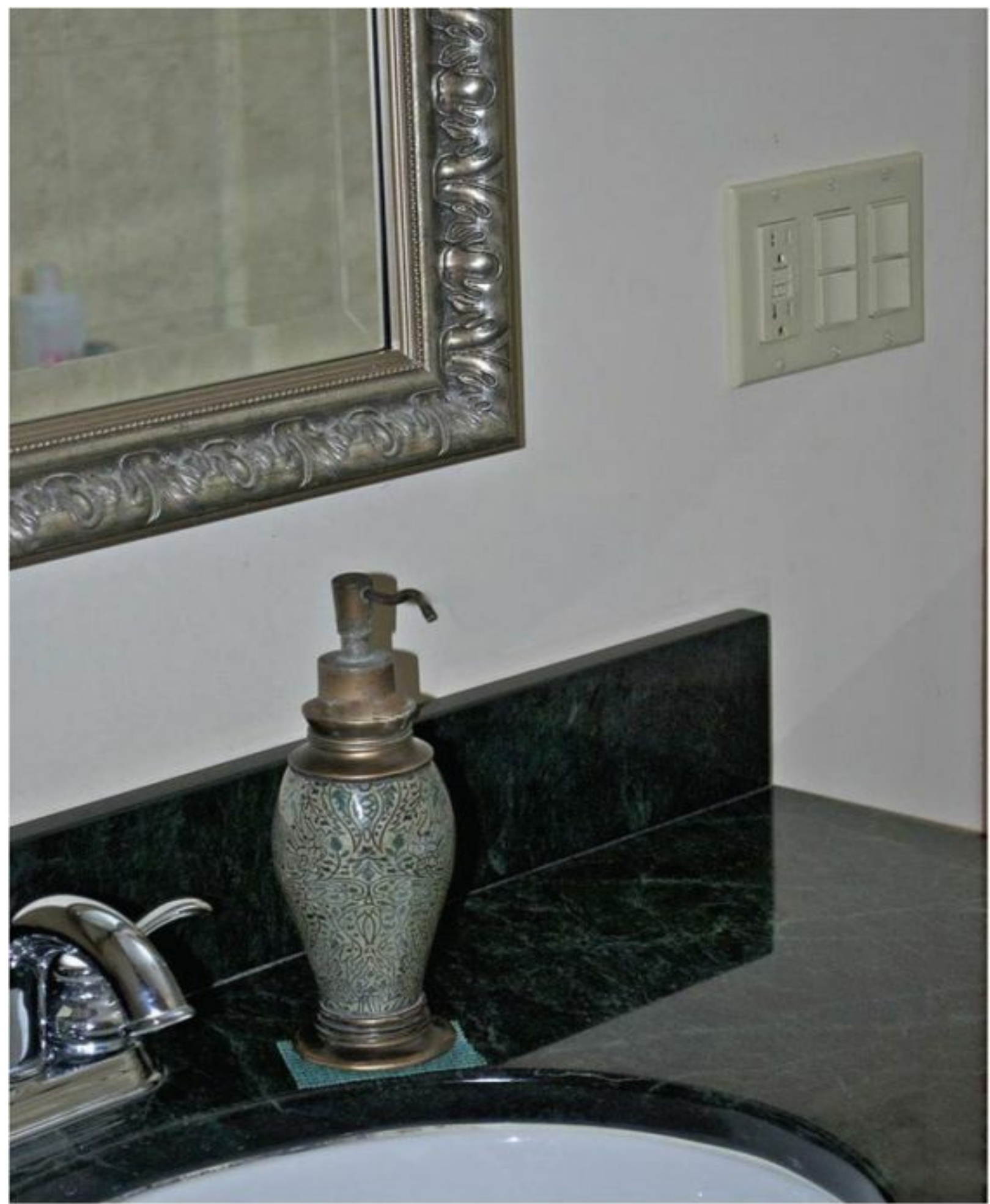
FIGURE G-19 Rocker switches combined with a ground-fault circuit interrupter (GFCI) are an attractive feature in this upscale bathroom.
