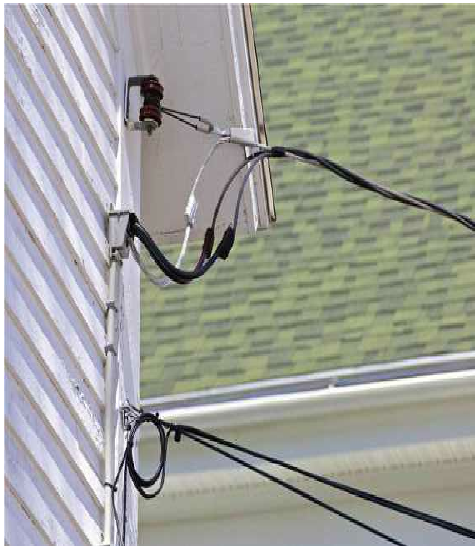
FIGURE G-18 Service drop with point of connection and weatherhead.
