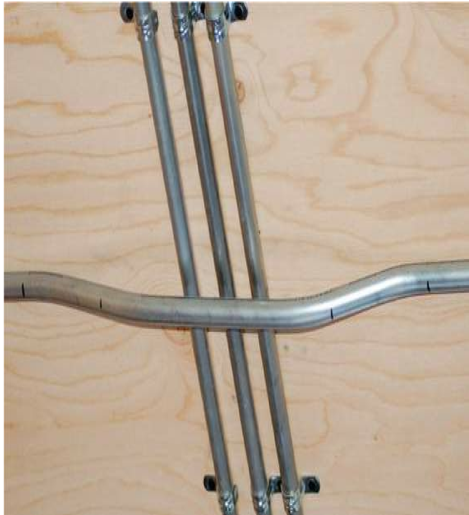
FIGURE 7-12 A two-point saddle bend, which is used where two or more pipes must be crossed.
