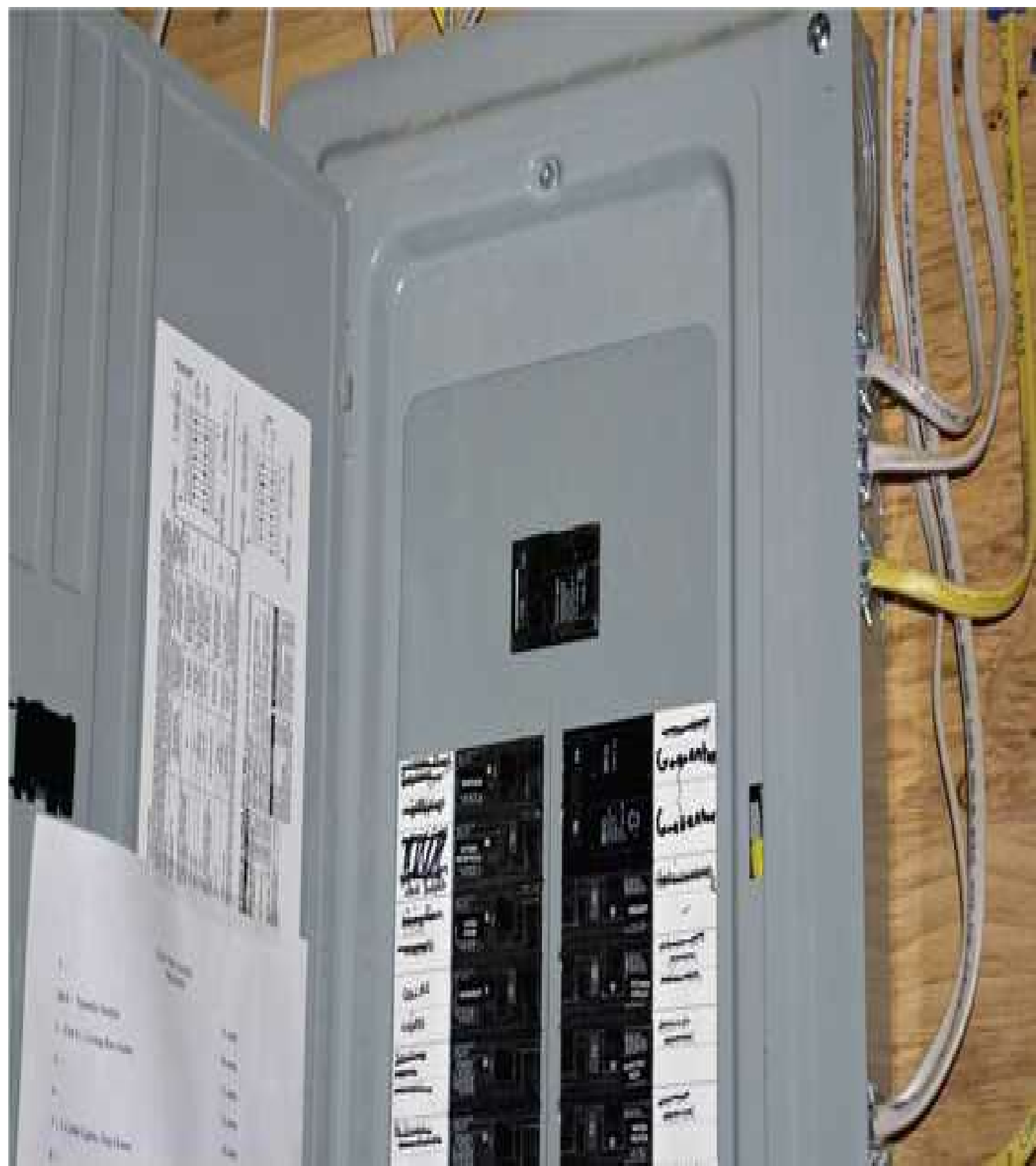
FIGURE G-12 The main disconnect is frequently located in the service-entrance panel.
