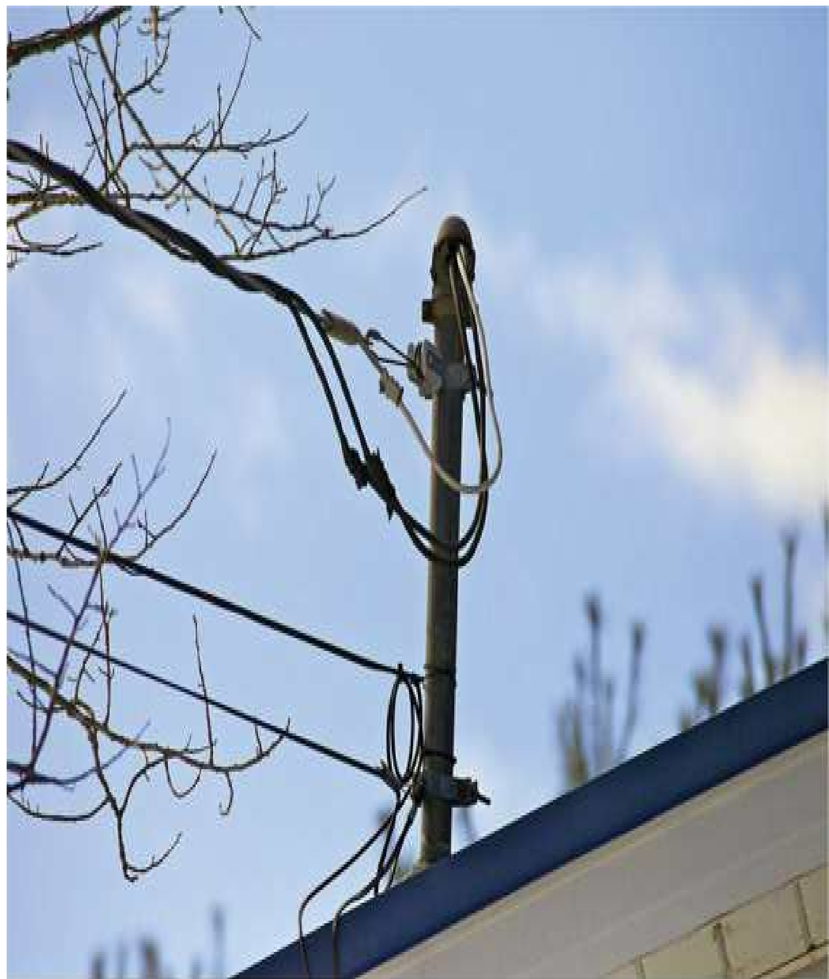
FIGURE 4-1 For this aerial masthead service, the point of connection consists of the crimped splices upstream from the weather head. (The cable TV and telephone cables attached to the service mast are a Code violation.)
