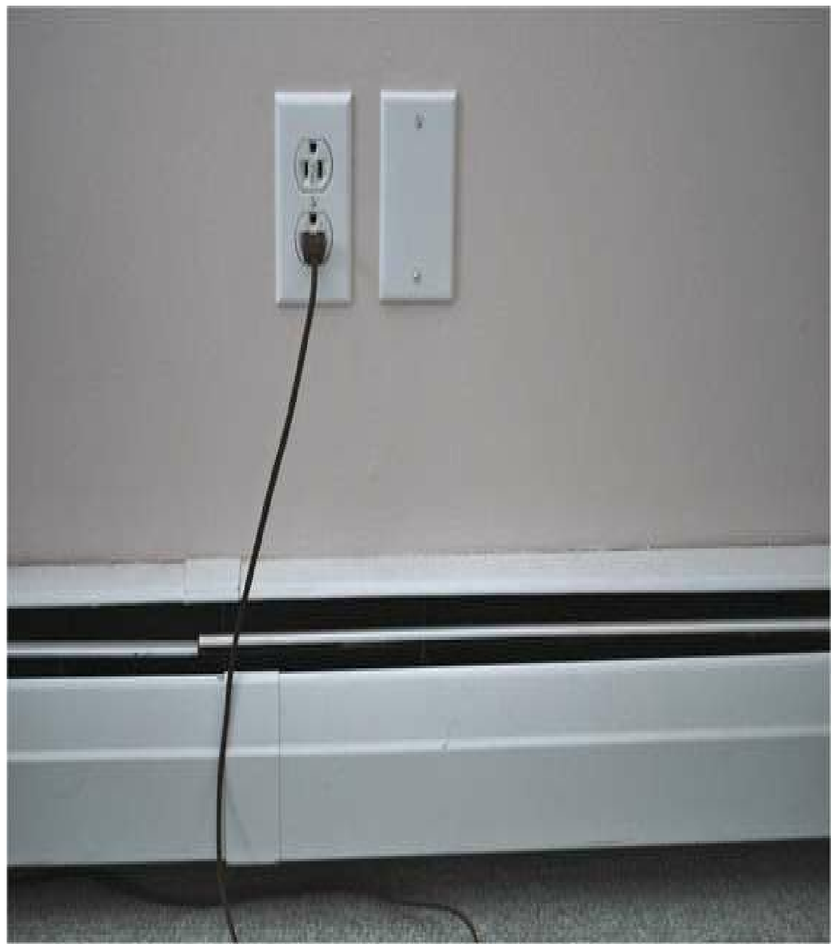
FIGURE 5-12 An electric baseboard space heater. The receptacle placed above it is a common listing violation because the cord is likely to enter the enclosure and be damaged by the heat.
