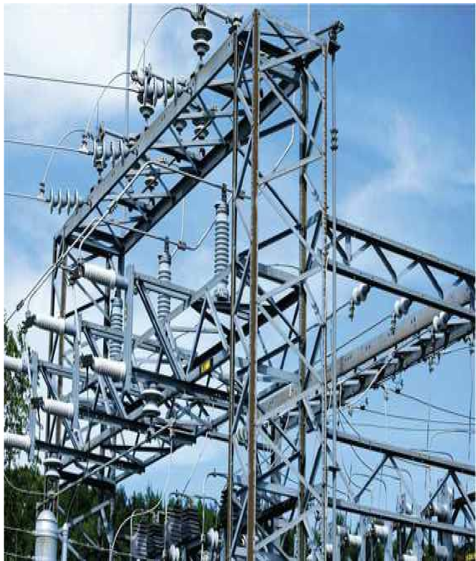
FIGURE 15-2 The substation is the source of local power, and the utility controls all lines that emanate from it.
