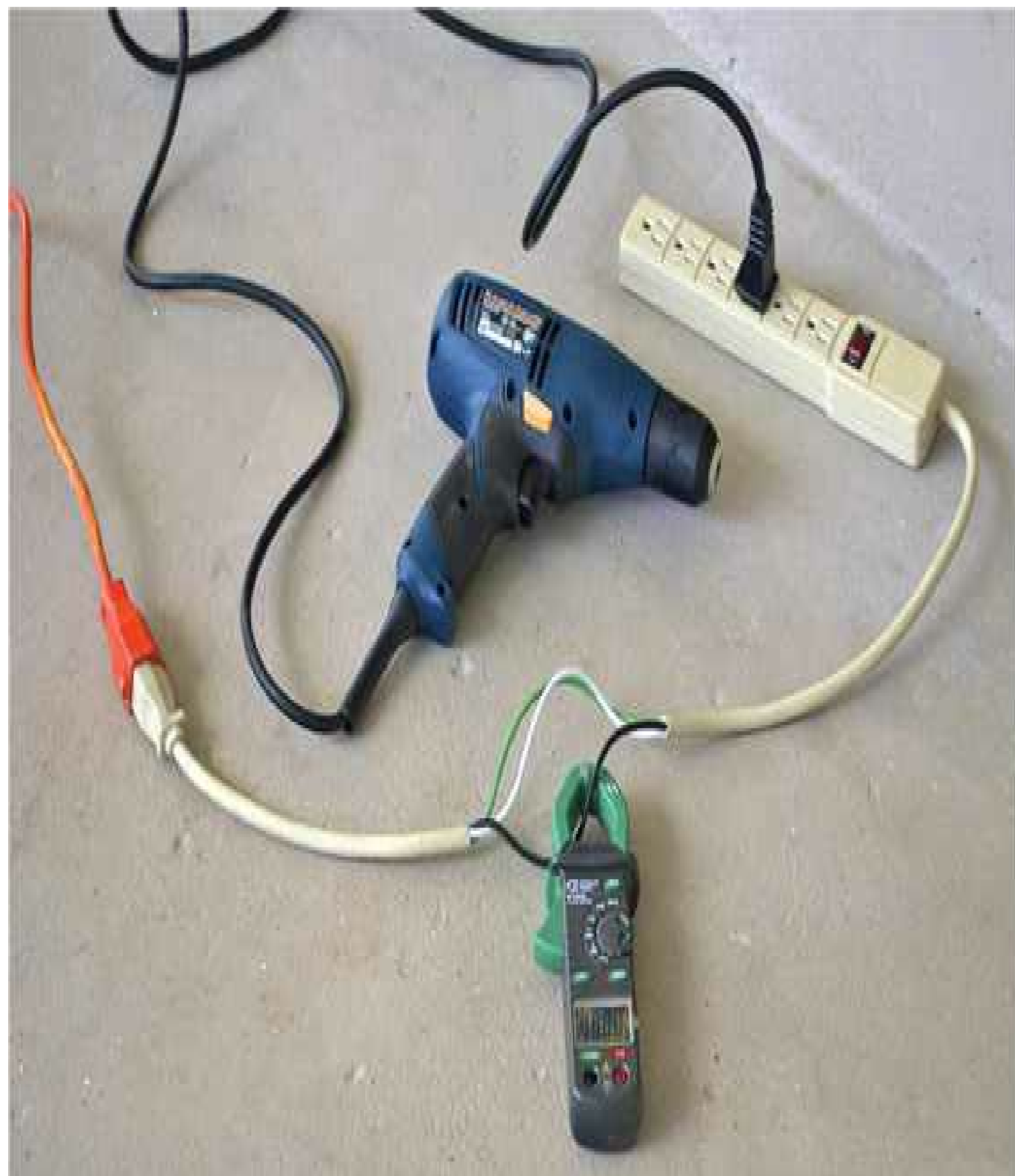
FIGURE 6-7 Clamp-on ammeter measuring current drawn by a portable power tool. Notice the homemade splitter, permitting reading a single conductor.
