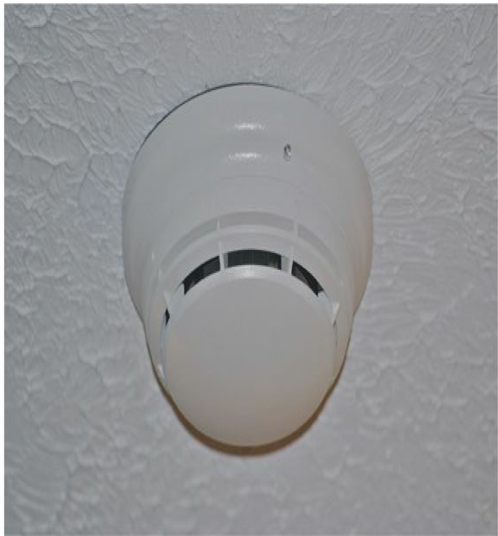
FIGURE 1-3 A smoke detector powered by a 9-volt battery and an ac branch circuit.
