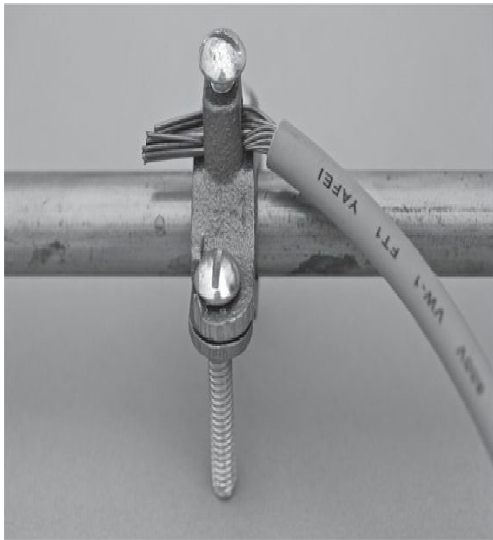
FIGURE G-9 Water pipe as a grounding electrode.
