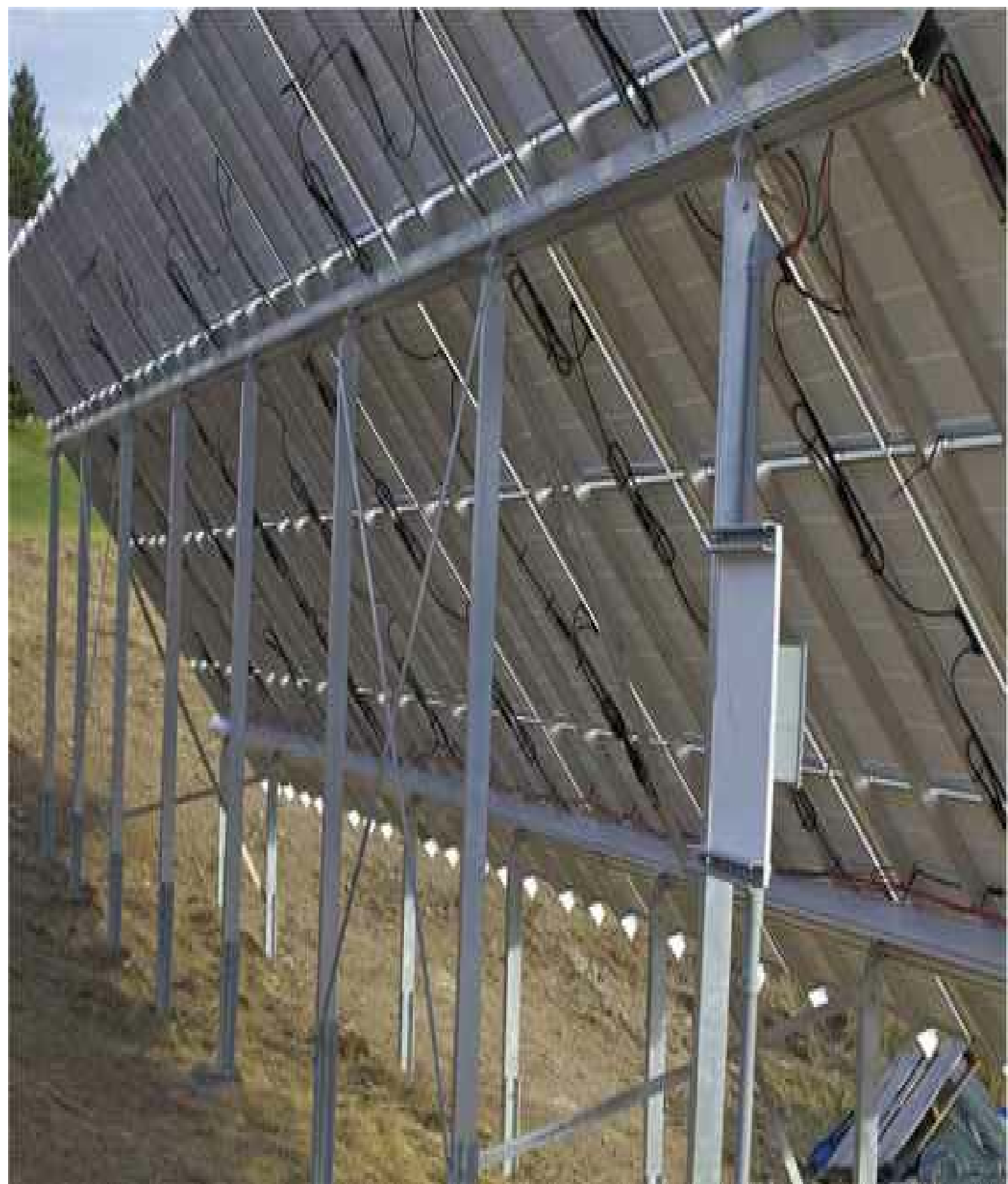
FIGURE 14-5 Sonotube concrete footings should not be too far out of the ground so as to limit pitting from the weather.
