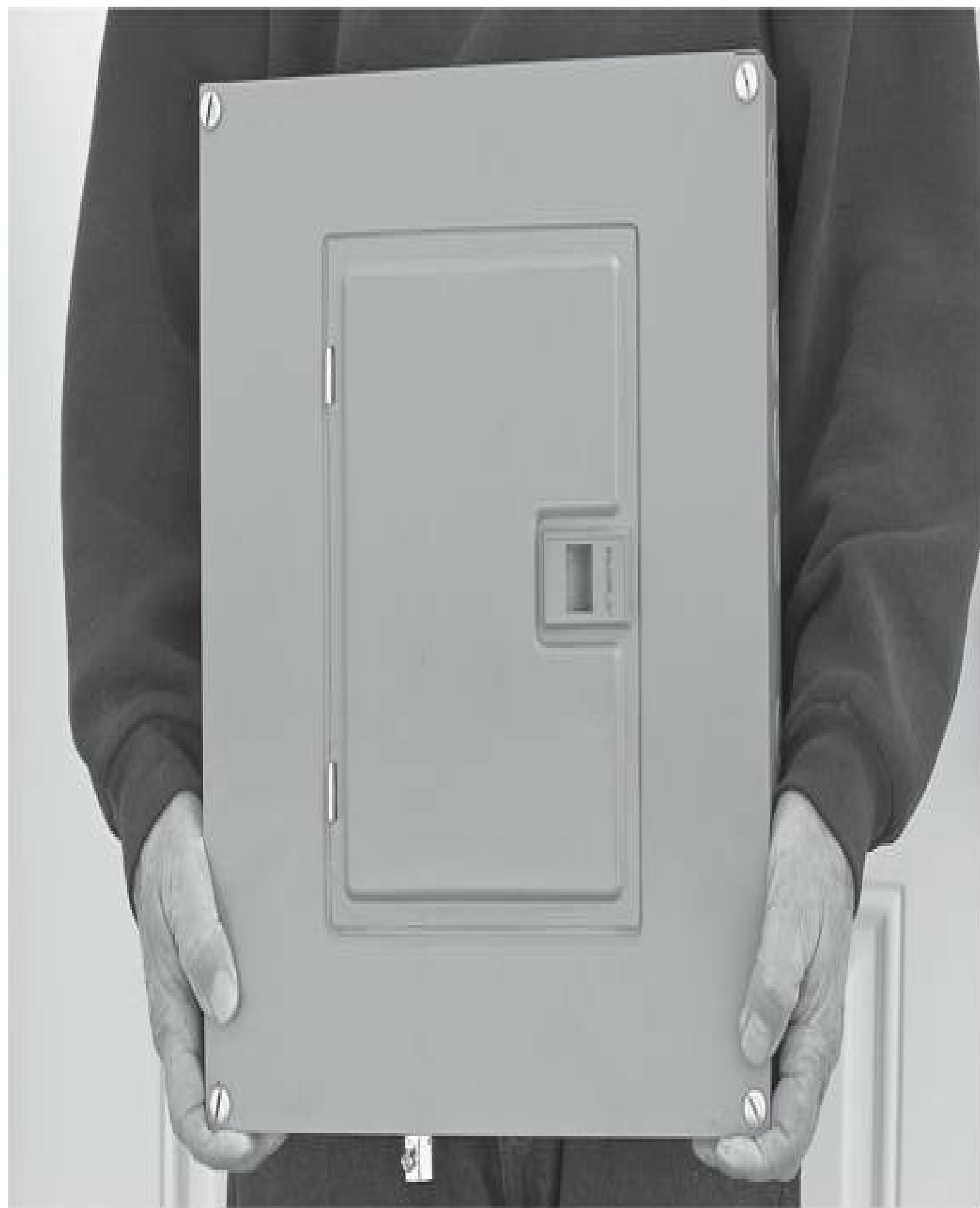
FIGURE 7-2 When designing a service, the location of the entrance panel must be considered.
