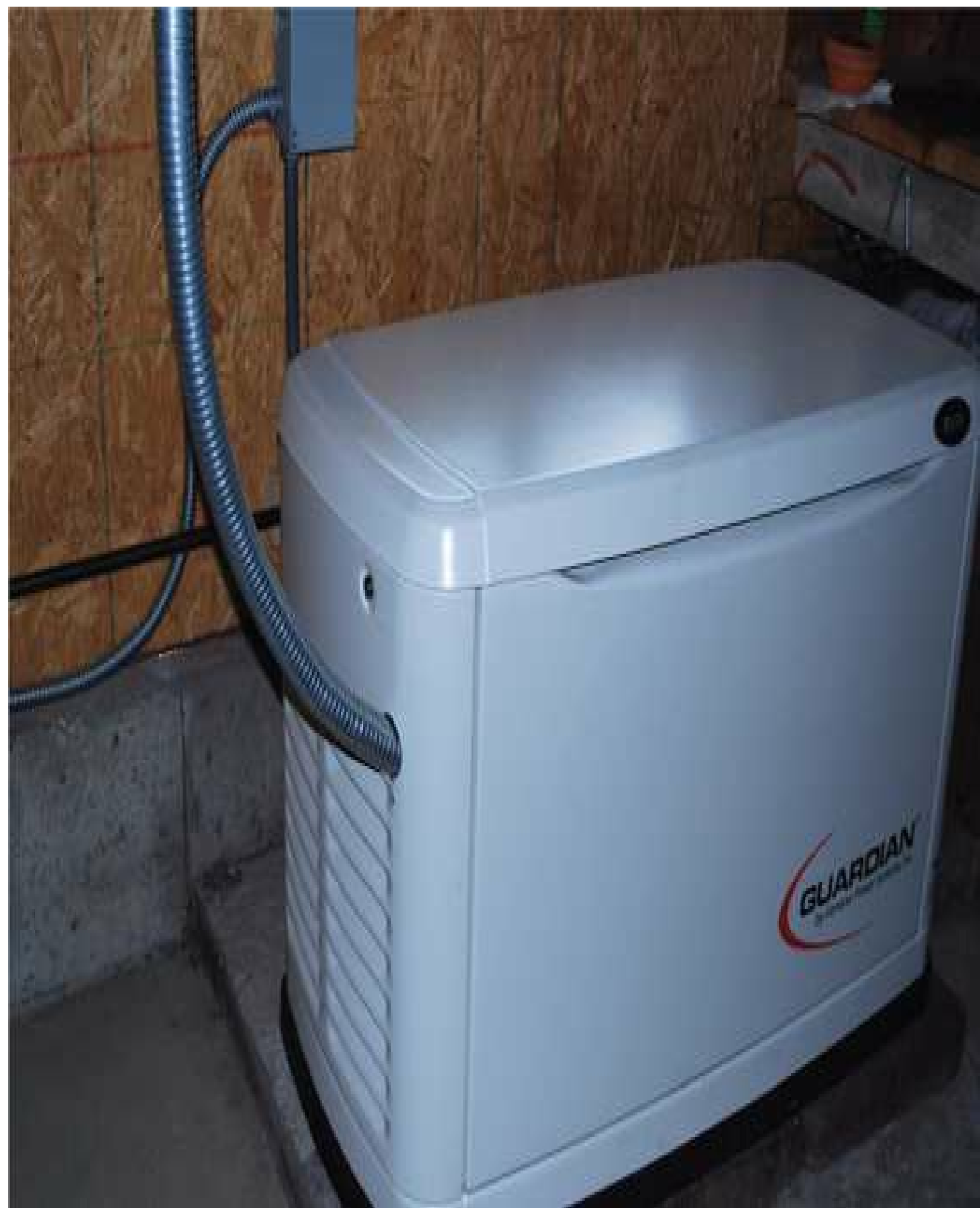
FIGURE 13-1 A small high-end generator.
