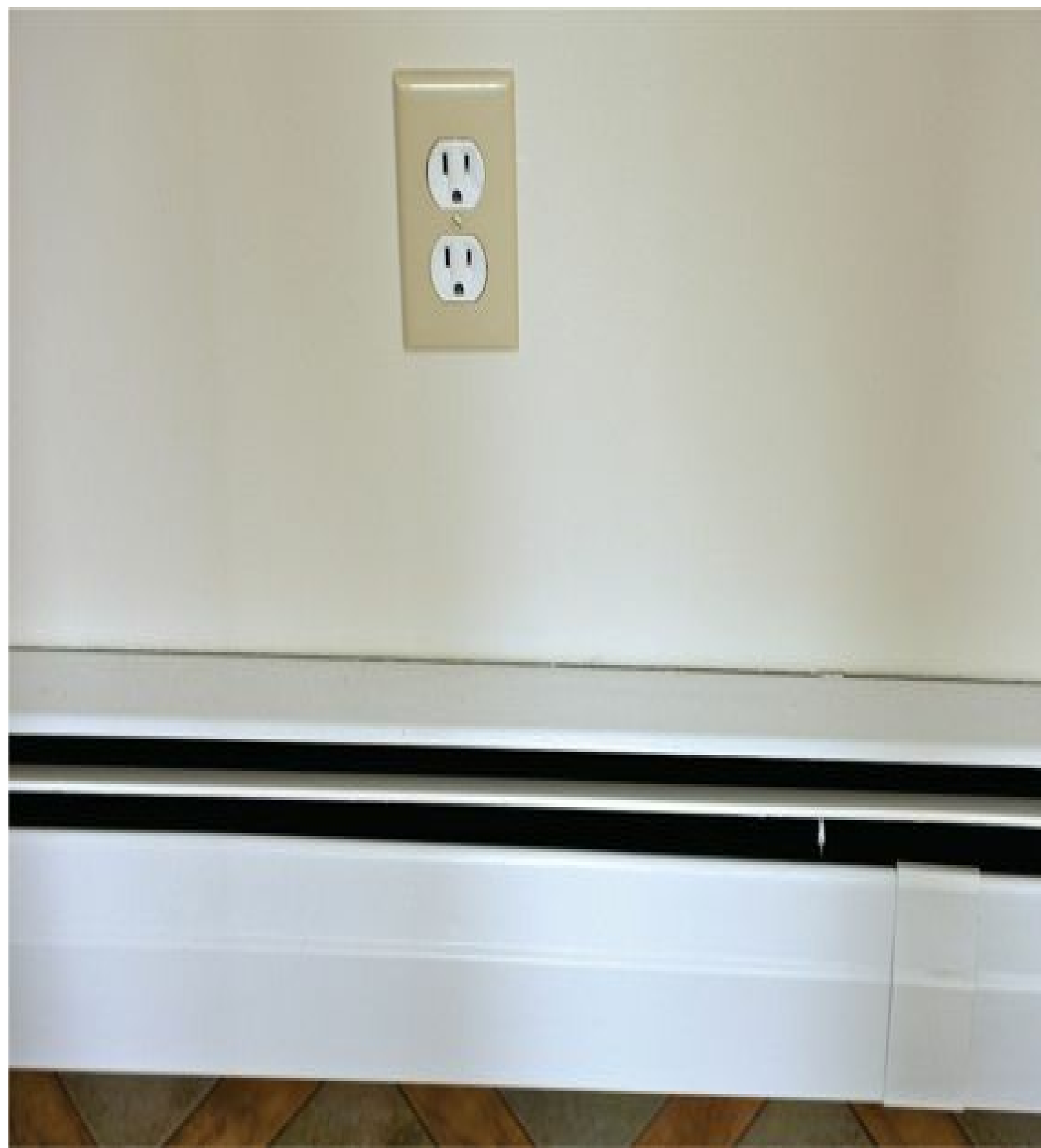
FIGURE G-16 This wall receptacle is improperly located above a baseboard heat unit.
