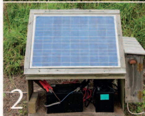
1. Our grid-linked wind turbine allows us to sell any excess electricity we create back to the national grid. 2. The energy created by these solar PV panels is stored in leisure batteries for such things as pumping water from our spring to powering our greenhouse heat sink.
