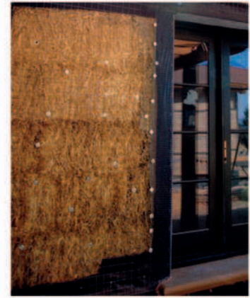
A wooden frame built with bale-sized spaces between the uprights is the perfect support.
