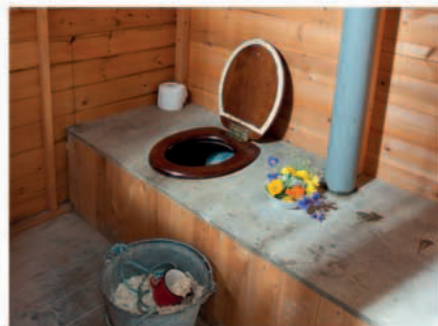
Instead of flushing sprinkle half a cup of sawdust down the loo and – very important – close the lid.
