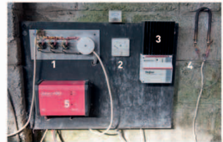
Converting water energy to electricity requires the following items: a rectifier (1), ammeter (2), charge controller (3), dump load (4), and pure sine inverter (5).
